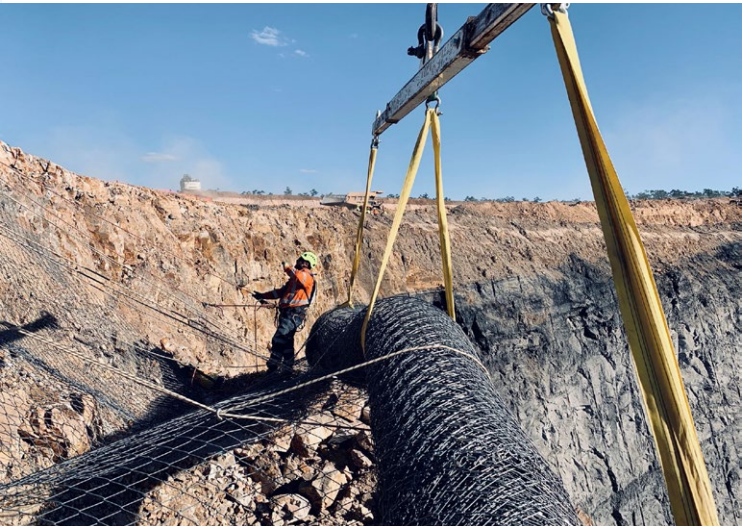
Middlemount Mine Rock Fall Protection
